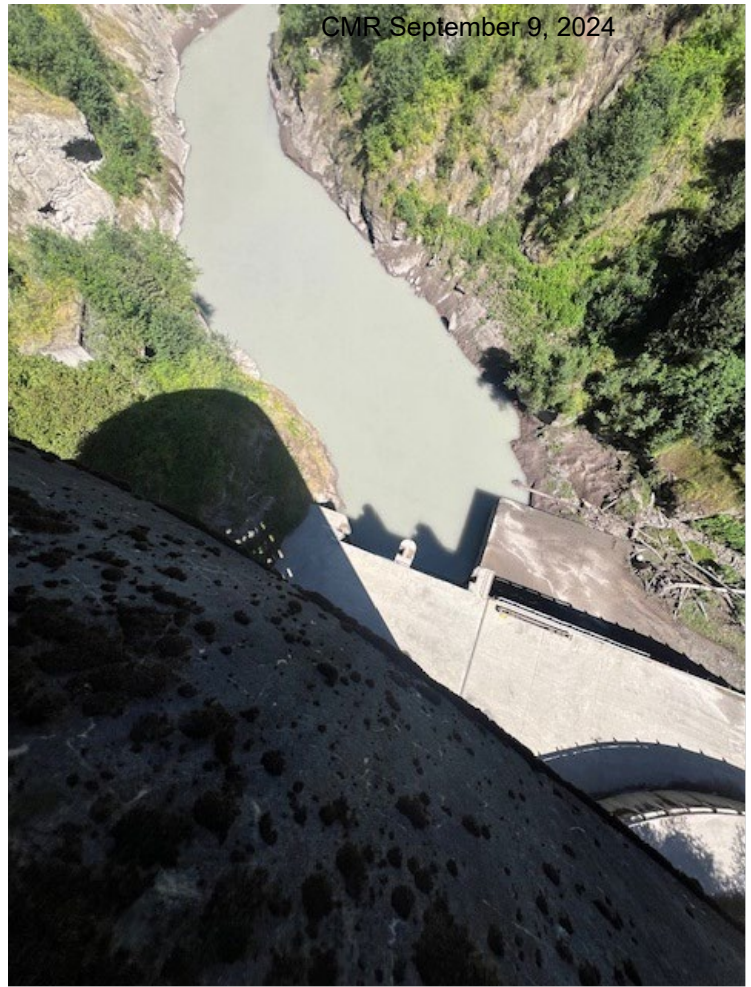
Looking down from the top of the cylindrical honeycomb water intake tower to the bottom stop-log gate where we were inside.
